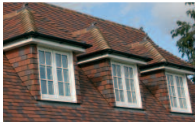
Above: An individual blend of Blue Brindle and Brown Antique tiles on a private house in Wiltshire.
