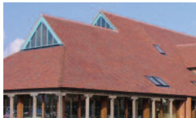
Above: The roof at Aston Pottery has a mixed blend of Red and Country Brown Tiles
