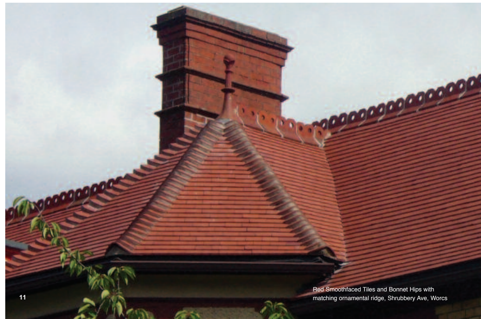
This Grade II listed Swiss style lodge, at Devonport Park, Plymouth, built in 1858, was refurbished with Red Dreadnought Ornamental Club tiles.
