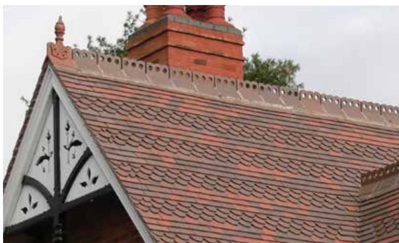
Above: This Victorian house was re-roofed using a mixture of brown brindle and country brown tiles with ornamental club tiles to match the original. Ornamental finials and ridge tiles were hand-made to match the originals.
