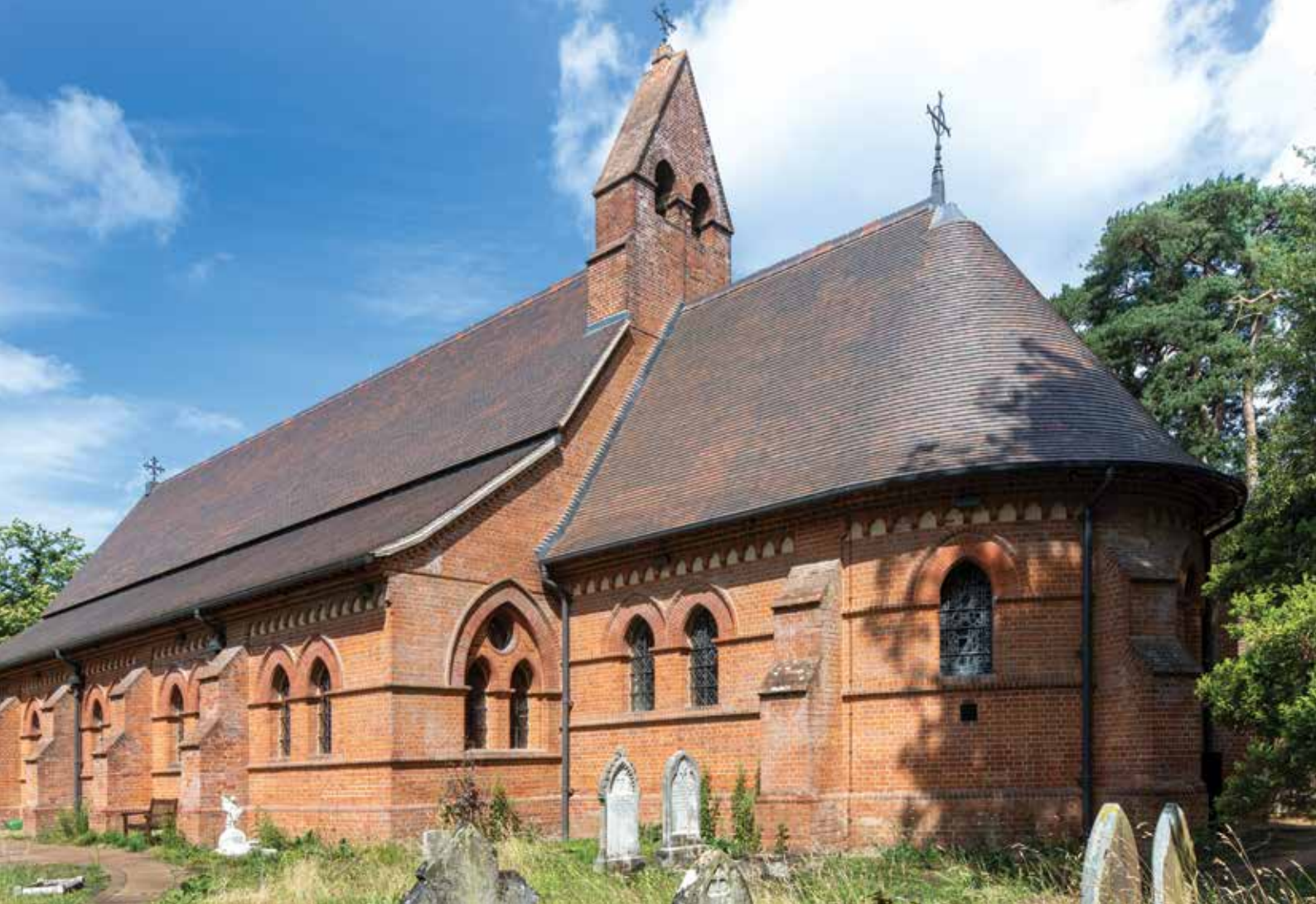
Above: Heritage architects Acanthus Clews specified Dreadnought brown brindle tiles and handmade cocks comb ridges after a devastating arson attack destroyed the existing roof and much of the interior of Grade II* listed All Saints Church in Fleet . The architects found these tiles provided the best match to the originals. The project was shortlisted for Best Heritage Roof at the 2023 Pitched Roofing Awards
